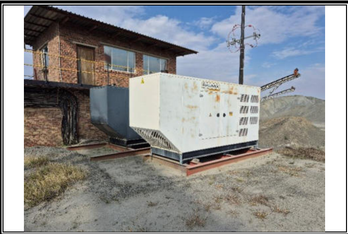
Bund walls to be added
