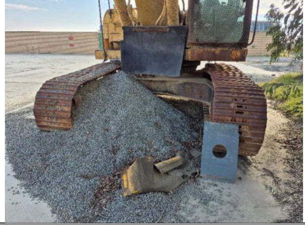
Old equipment to be removed from site
